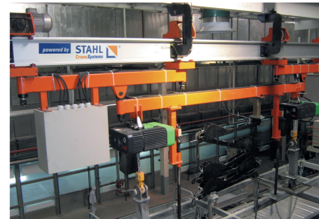
In a coating plant for the automotive industry in China, 48 specially designed ST chain hoists operate at very high humidity levels.
